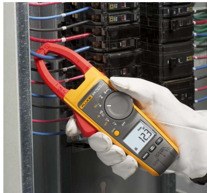
Measuring current with a clamp meter.
